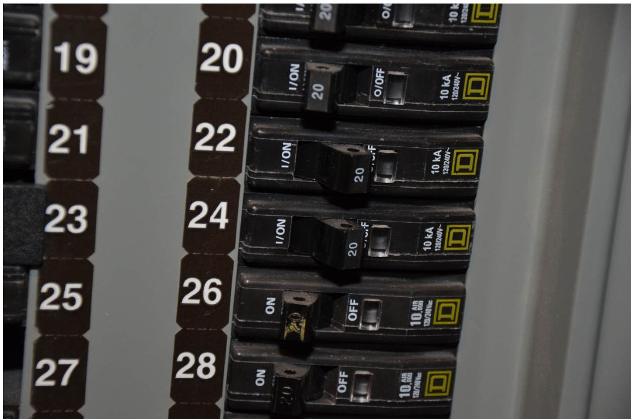
Circuit Breaker Panelboard.
